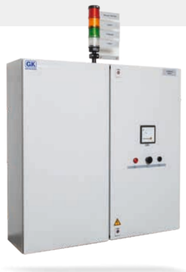
PDU (Power distribution unit)
