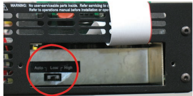
Figure 5.12 – Bi-Level Power Switch Location
